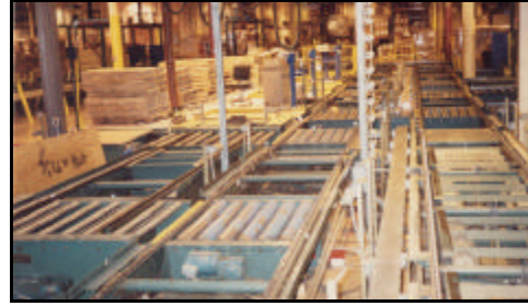
Schering Plough, NJ – More than ½ of the conveyor pictured here, was removed.
